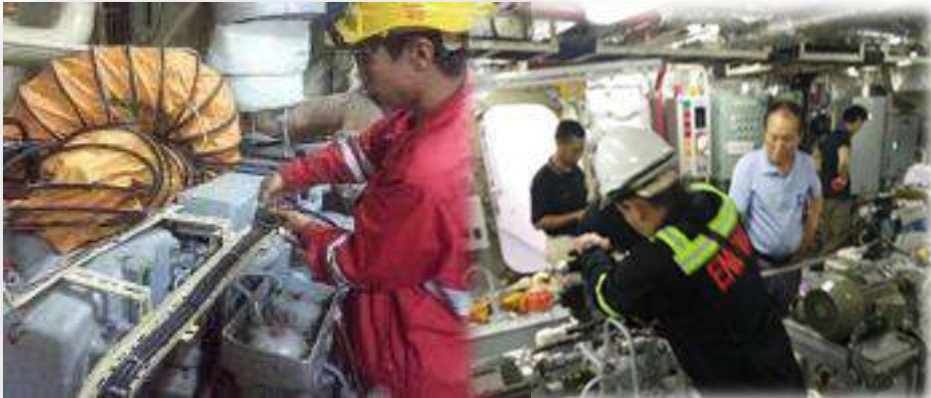
Ship Lighting Distribution Box and Controllers Servicing & Test
