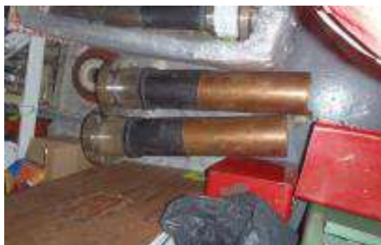
CATHODIC PROTECTION ZINC ANODES
