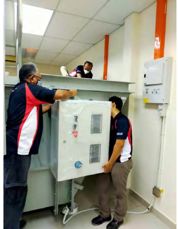
CONTROL PANEL INSTALLATION
