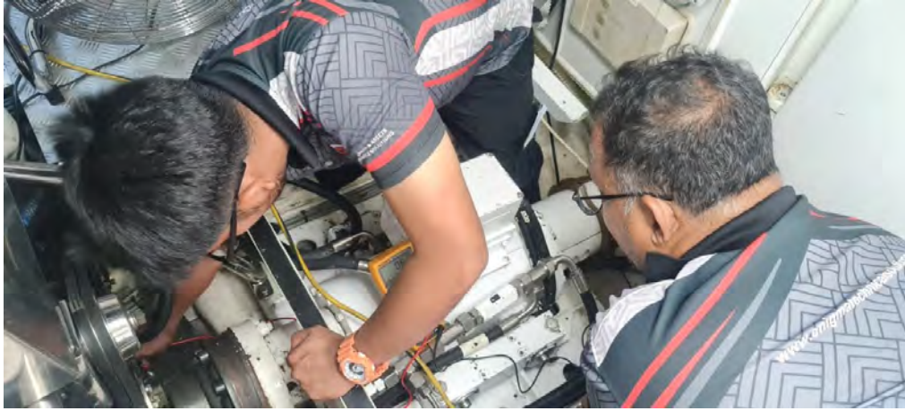
CHECK FOR SHAFT EARTHING
